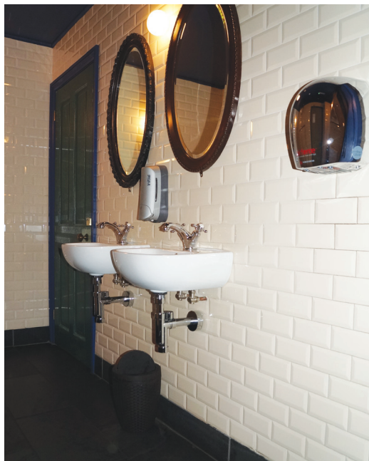
The water from the sinks in the ladies bathroom is also discharged through small bore pipework in to the XL.
