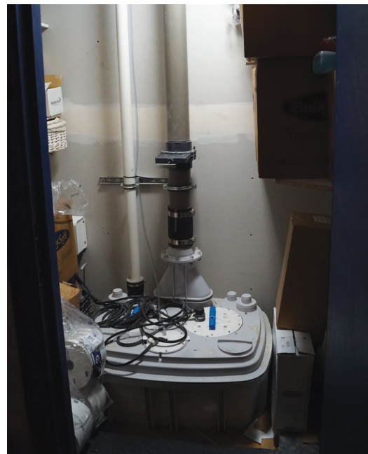
The Sanicubic XL has been installed in a cupboard which keeps it out of sight, eliminates any noise but is accessible for maintenance.
