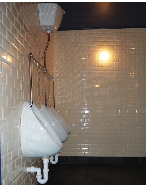
The waste from the men's bathroom is pumped up to a Sanicubic XL located in a cleaners cupboard.
