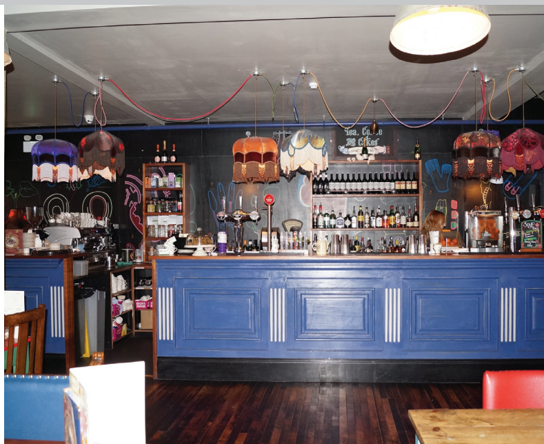
The bar is positioned away from the back wall and drainage is only possible thanks to the Sanicom with small bore pipework.
