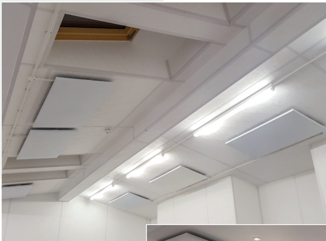
RP radiant panels ceiling mounted in a cricket pavilion
