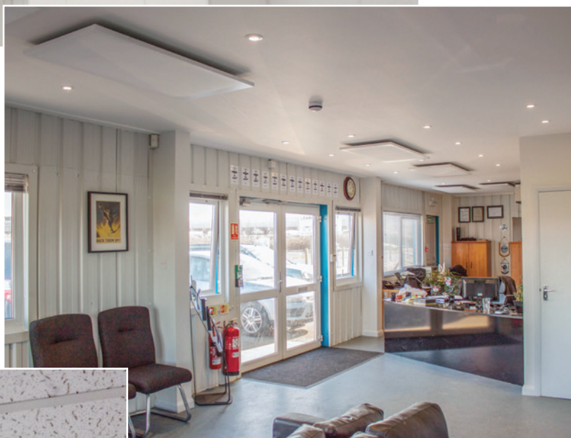
RP-06 Radiant Panels providing an economic and stylish means of heating a flying school in Sussex
