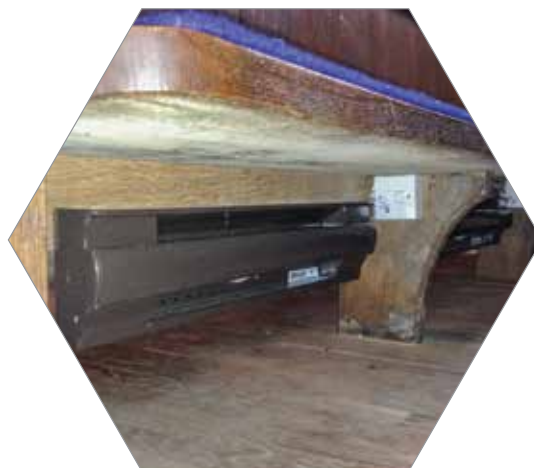
BLC heaters installed under pews in St Bartholomew's Church Notgrove
