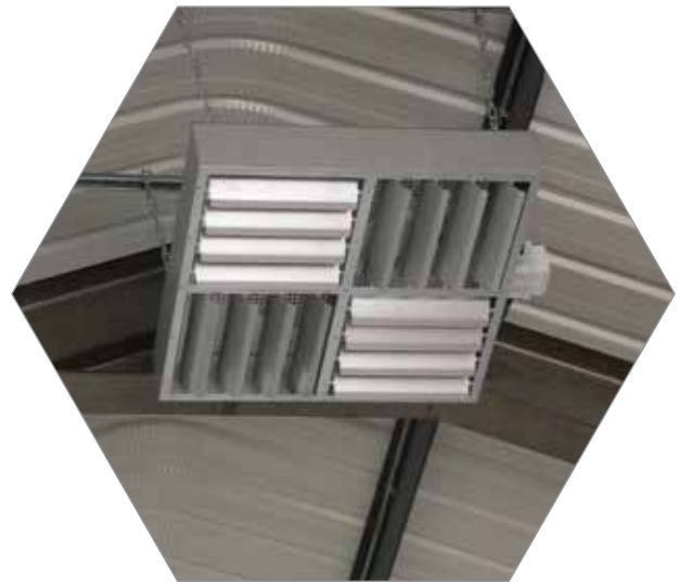
DSU-4 installed in a vehicle repair shop in Kent
