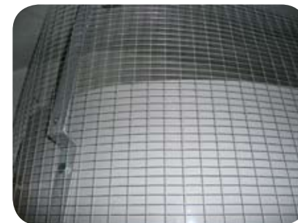
Bird Guard installed in RCF Roof Cowl
